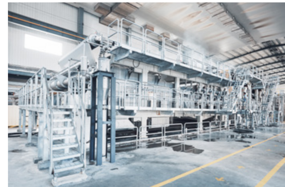
The pulp drying line consists of a TwinWirePress pulp machine, airborne dryer, cutter-layboy, and bale finishing system.
